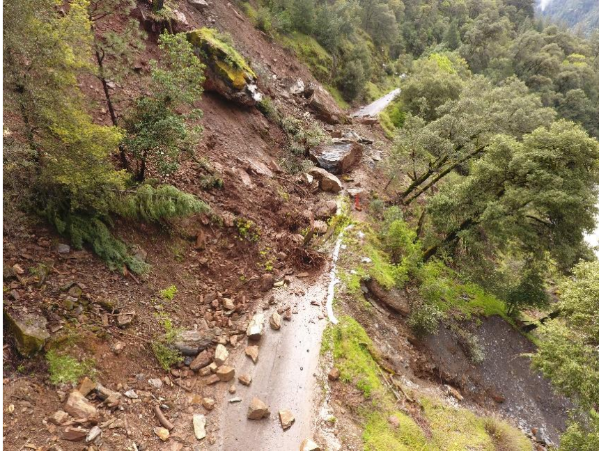
Figure R-9 Blacksmith Flat Road Landslide 2017
