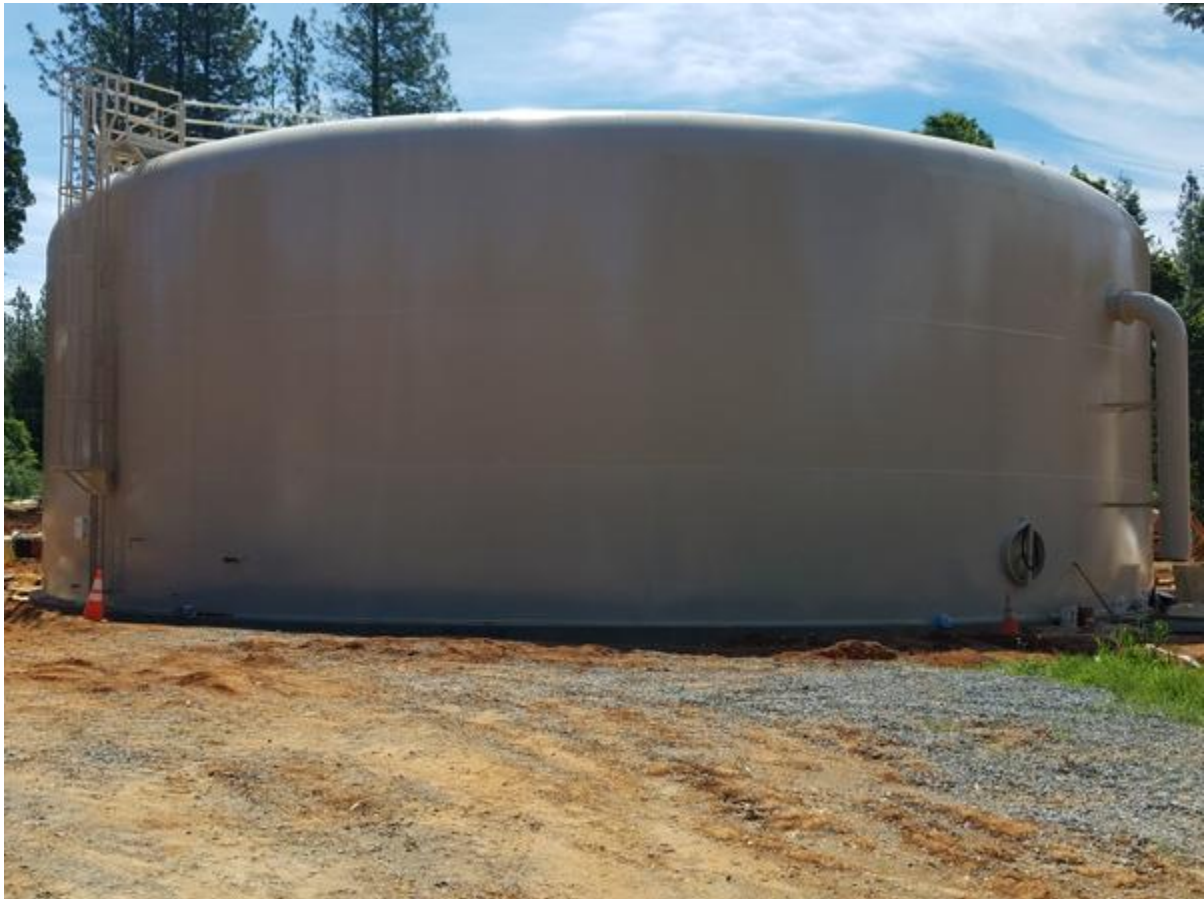
Figure I-5 Water Storage Tank
