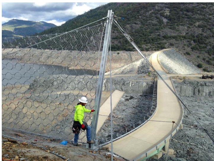
Figure R-8 Rockfall Netting Above Hell Hole 2016
