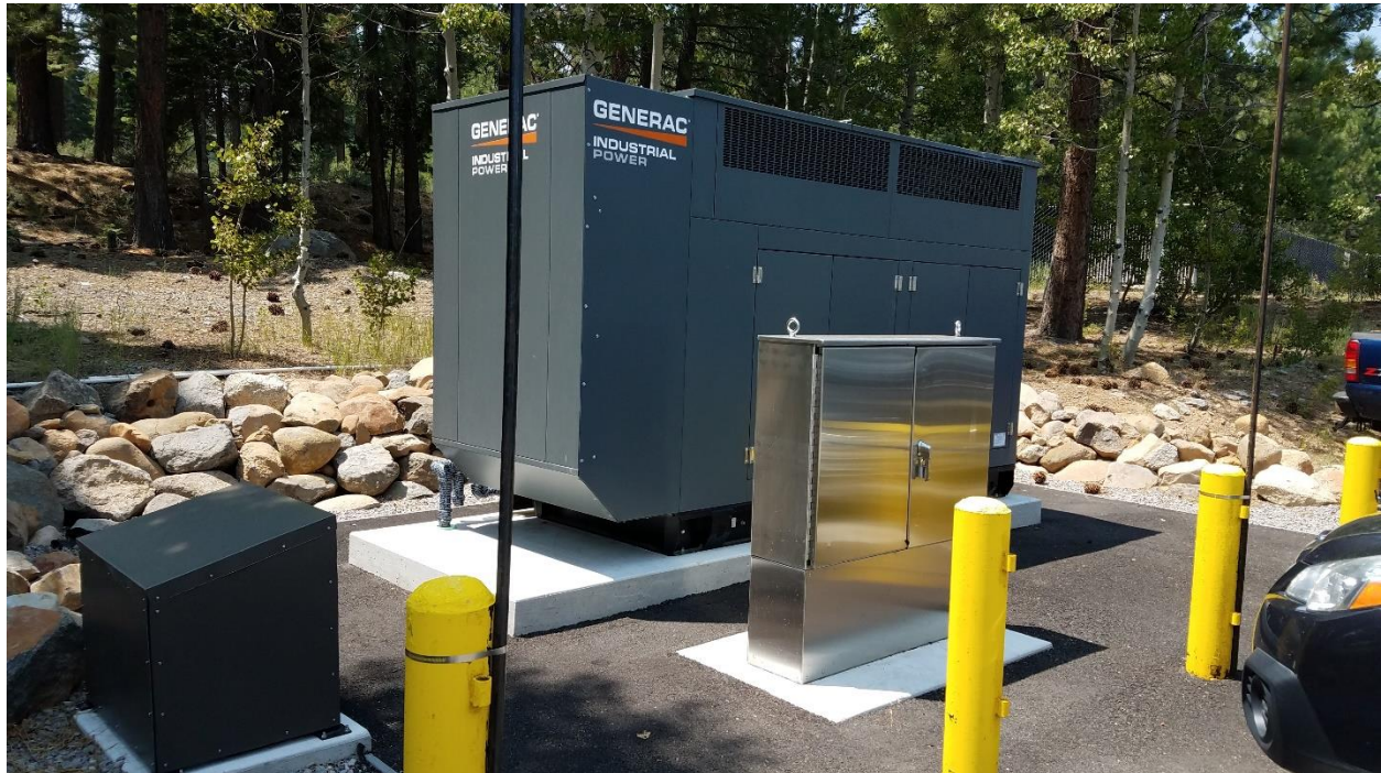
Figure 2-2 North Tahoe Public Utility District Generator
